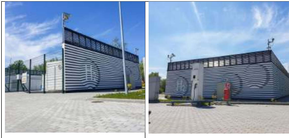
Figure 15. Riga Hydrogen production and refuelling station
